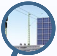
Cables for catenary
