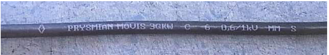
CABLE MARKING : meter marking 56811 PRYSMIAN MOVIS 3 GKW C 6 0,6/1KV MM S
